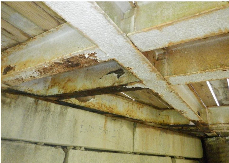
FB 1/2- PC FAILURE/CORROSION THROUGHOUT FB 1/2 BTW STR 1-4
