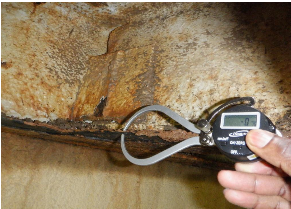
STR 1 @ END BENT 1 1/16" REMAINING BOTTOM FLANGE 2' SEGMENT
