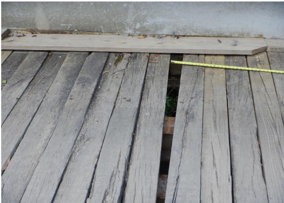
4" GAP IN DECKING OVER FLOORBEAM 6
