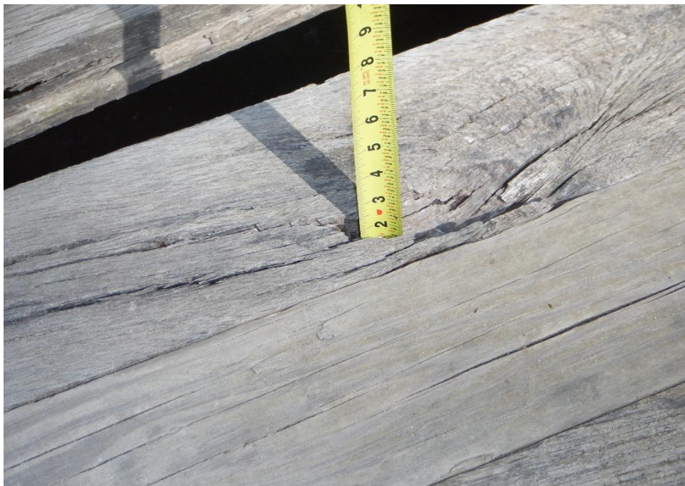
2" DEEP AREA OF DECAY IN DECKING BTW FLOORBEAM 5/6
