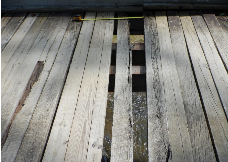
MISSING DECKING BTW FLOORBEAM 5/6
