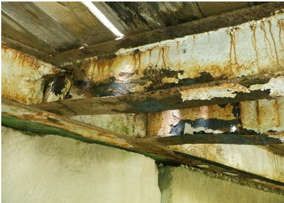
STR 1 - 16"X8" HOLE IN WEB; BUCKLING AT FB 9 JUNCTION - PAR 3/8" REMAINING TO BOTTOM FLANGE
