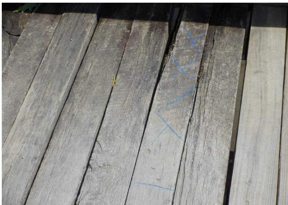
3' L DECAY IN DECK BOARD BTW FLOORBEAM 6/7- NORTH SIDE
