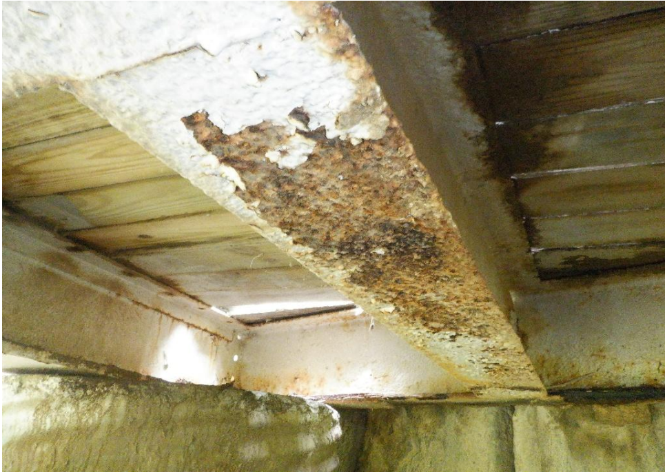
STR 4 1/8 DEEP PITTING BOTTOM FLANGE 4' SEGMENT BTW FB 1/2
