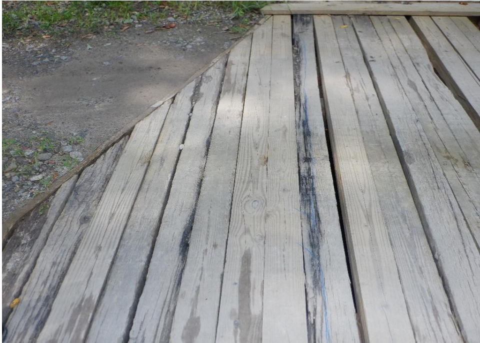
9' L AREA DECAY AT END BENT 2 BTW FLOORBEAMS 8/9
