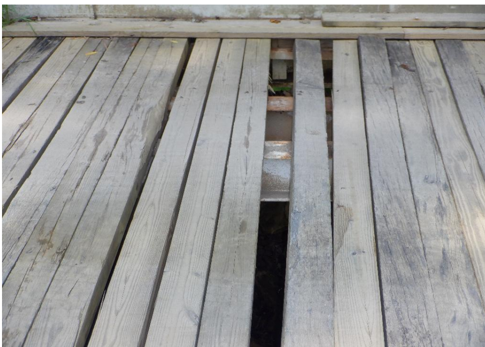
MISSING DECKING BTW FLOORBEAM 7/8 AT FLOORBEAM 8
