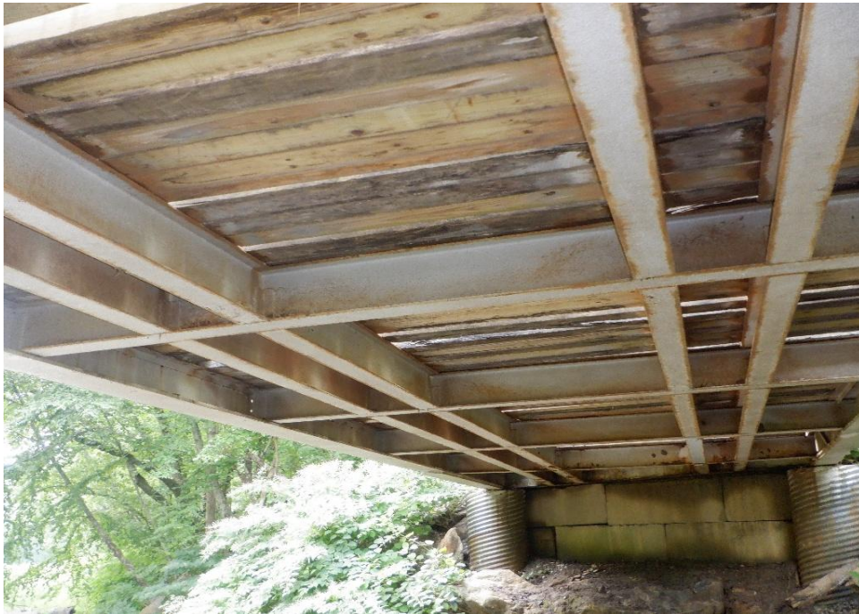
FB 5- PC FAILURE THROUGHOUT W/ CORROSION PRESENT
