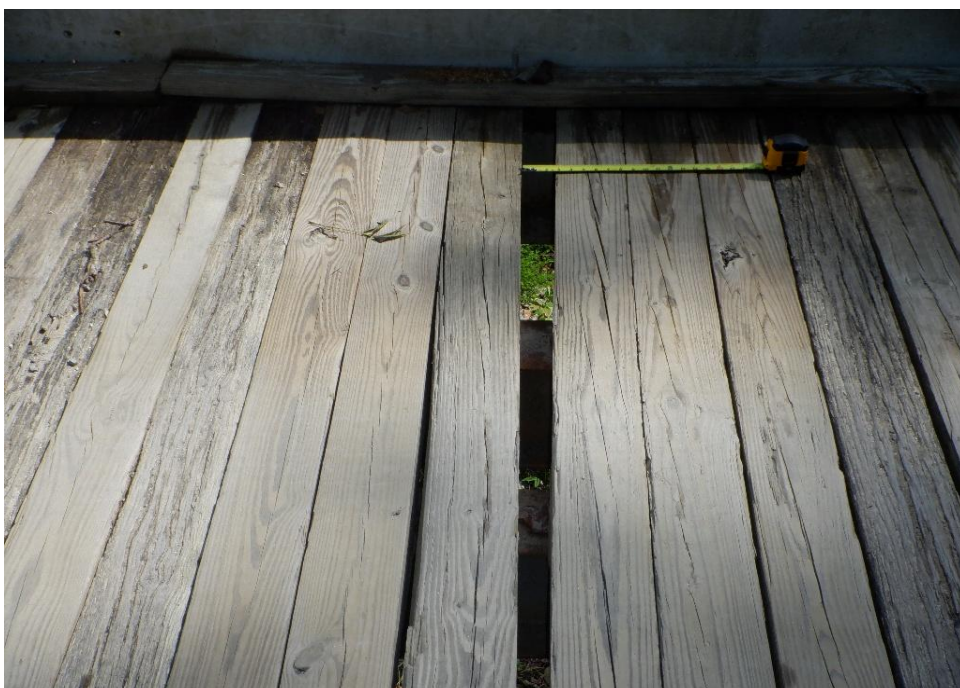
3" GAP IN DECKING BTW FLOORBEAMS 3/4
