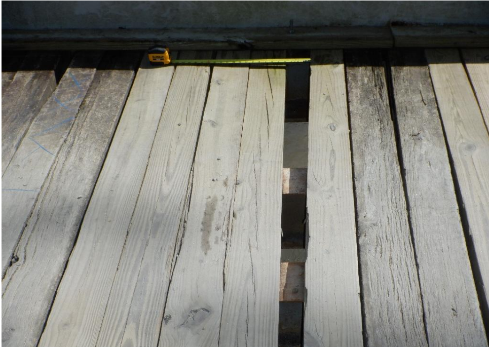
4" GAP IN DECKING BTW FLOORBEAM 6/7
