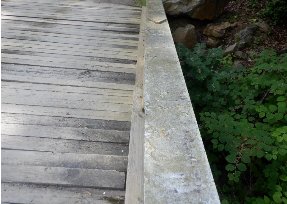
PROTECTIVE COATING FAILURE THROUGHOUT TOP FLANGE GIRDER 2
