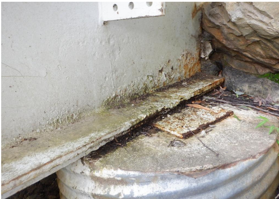
EB 2 GIRDER 2 BEARING/WEB PC FAILURE & CORROSION PRESENT
