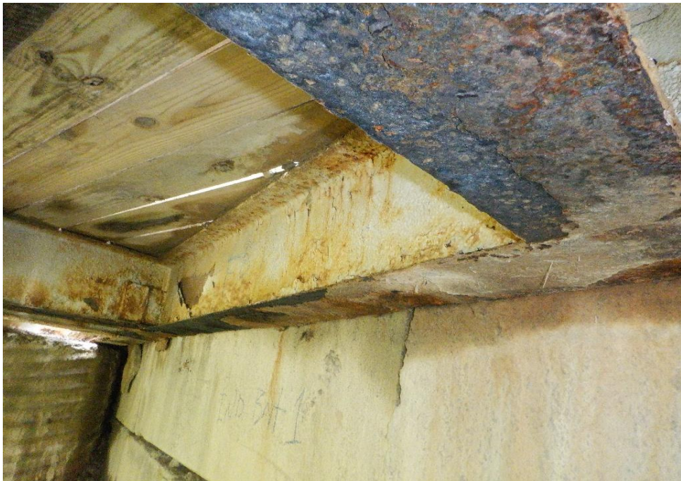
ALT. VIEW- 7/32" REMAINING BOTTOM FLANGE FLOORBEAM 1
