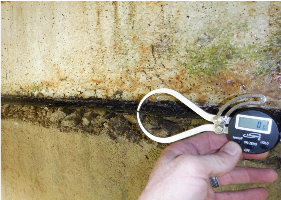
FB 9 3/64" REMAINING TO BOTTOM FLANGE FULL LENGTH
