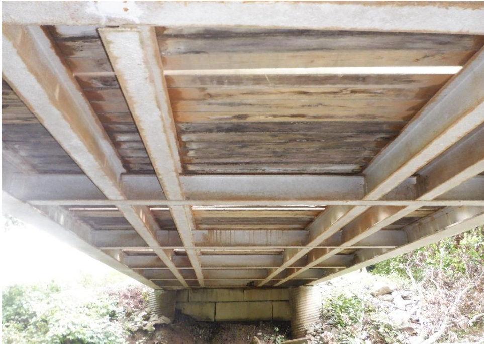
FB 6 - PC FAILURE THROUGHOUT W/ CORROSION PRESENT
