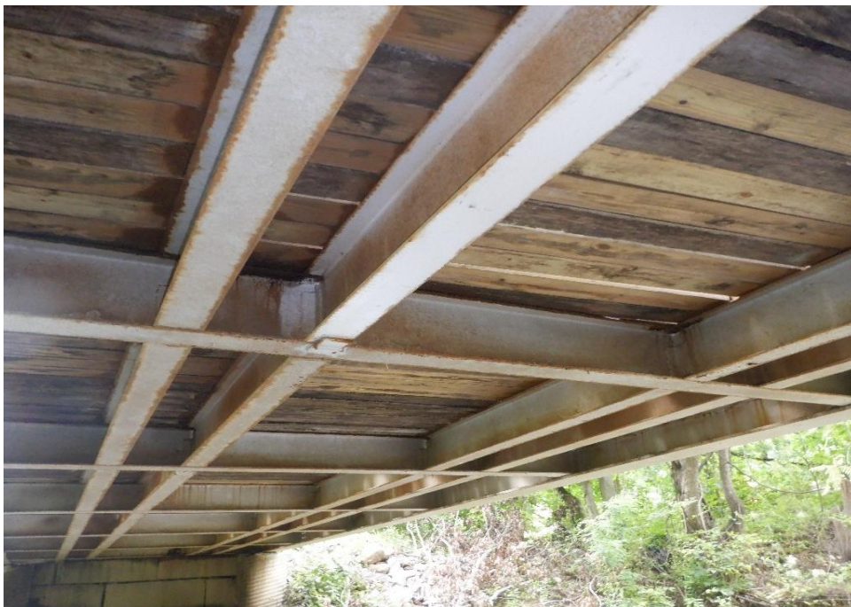
FB 7 PC FAILURE THROUGHOUT W/ CORROSION PRESENT
