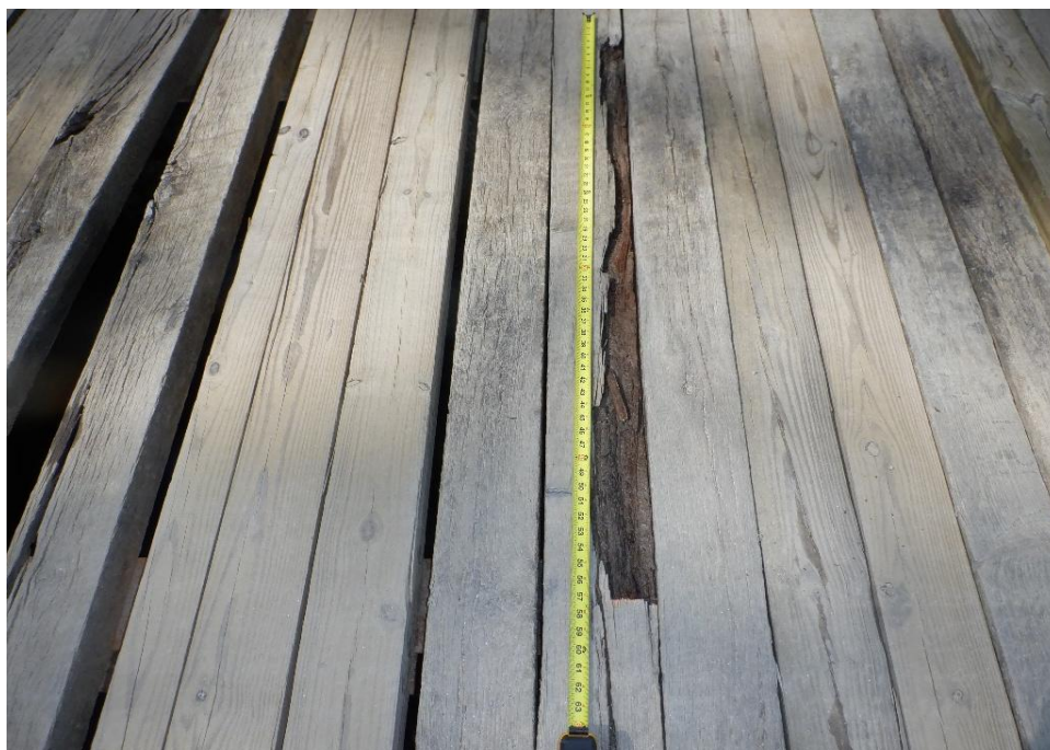
5' AREA OF DECAY IN DECKING BTW FLOORBEAM 5/6
