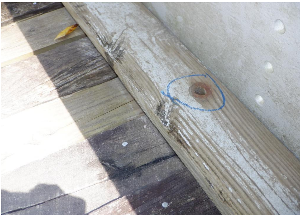
1 MISSING BOLT @ WHEEL GUARD N. SIDE AT FLOORBEAM 6
