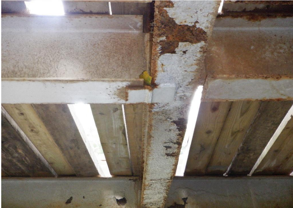
FB 8 ACTIVE CORROSION W/ 1/8" PITTING FULL LENGTH
