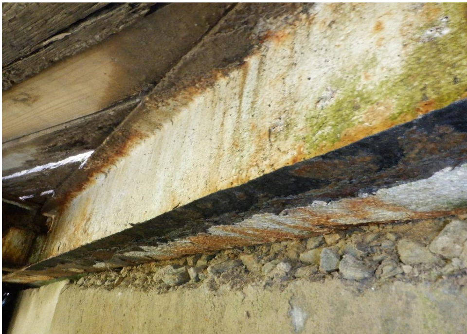
FB 9 OVERVIEW BOTTOM FLANGE 3/64" REMAINING
