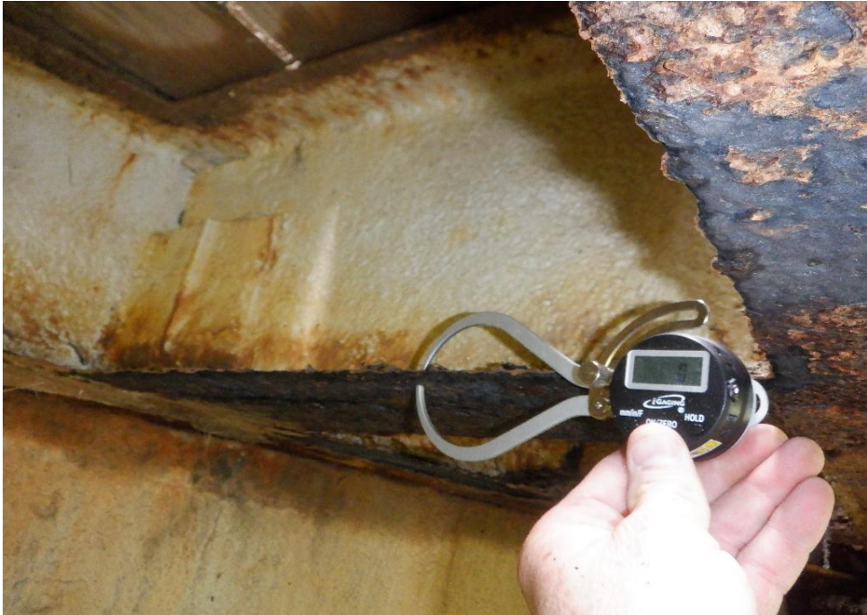
STR 2 @ END BENT 1- 1/64" REMAINING 2' SEGMENT BOTTOM FLANGE
