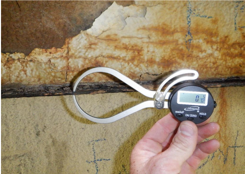
FLOORBEAM 1- 7/32" REMAINING 10' SECTION BOTTOM FLANGE
