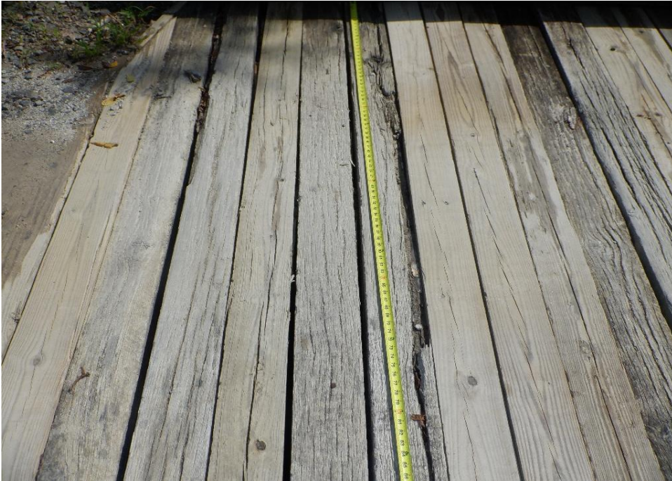
10' L AREA OF DECAY IN DECKING OVER END BENT 1
