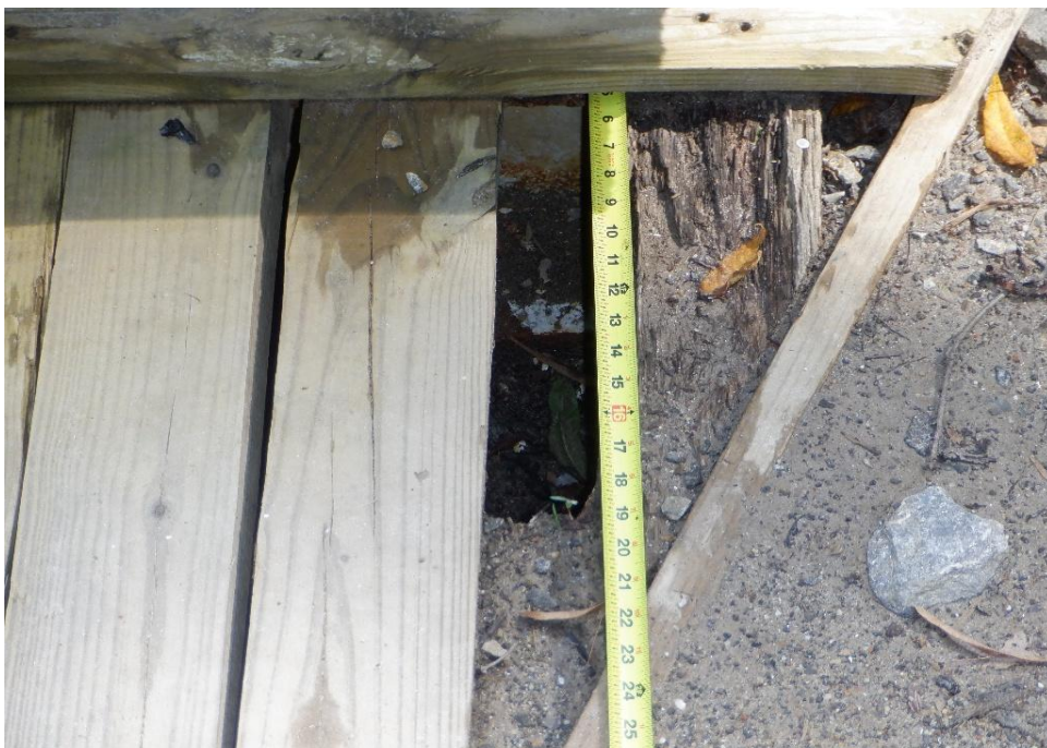
2' L AREA DECAY IN DECKING N. SIDE OVER END BENT 2
