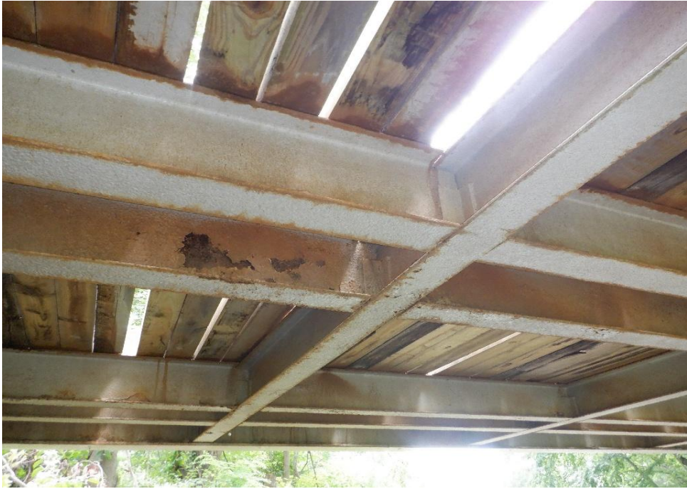
FB 3- RUST/BLEED THROUGH - PC FAILURE W/ CORROSION PRESENT
