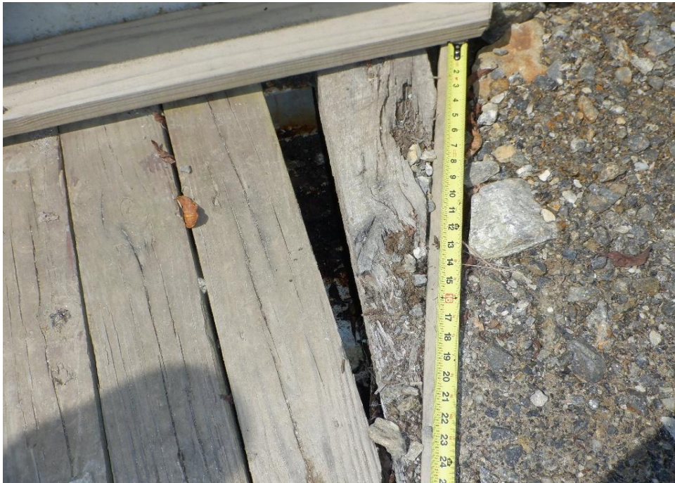
2' AREA DECAY IN DECKING OVER END BENT 1 SOUTH SIDE
