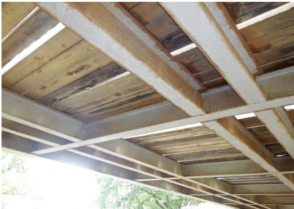
FB 4- PC FAILURE THROUGHOUT W/ CORROSION PRESENT
