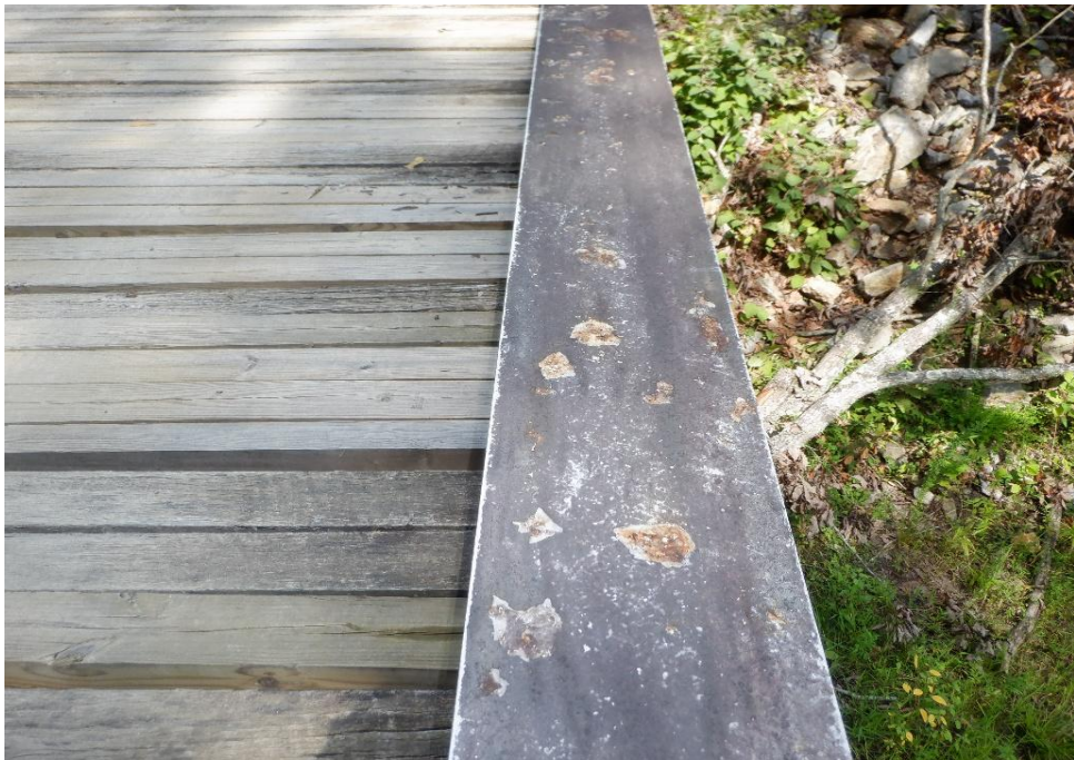
PROTECTIVE COATING FAILURE THROUGHOUT TOP FLANGE GIRDER 1
