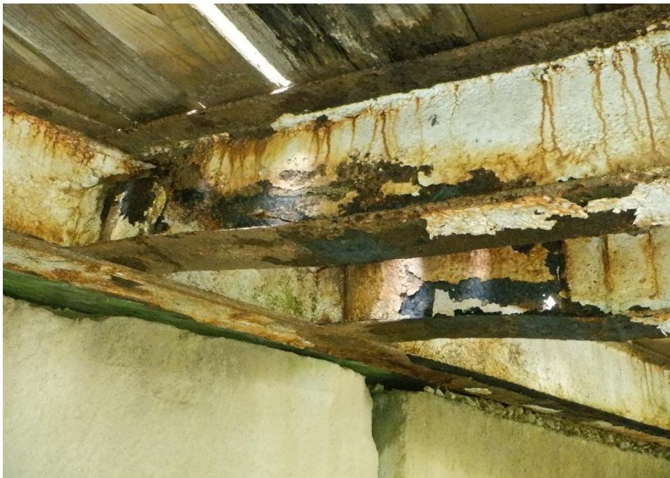
ALT. VIEW-STR 2 - 1'X10" HOLE IN WEB; BUCKLING AT FB 9 JUNCTION - PAR 5/16" REMAINING TO BOTTOM FLANGE
