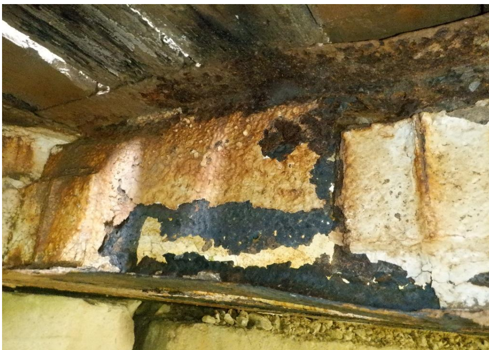
STR 2 - 1'X10" HOLE IN WEB; BUCKLING AT FB 9 JUNCTION - PAR 5/16" REMAINING TO BOTTOM FLANGE
