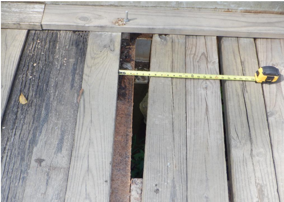
5.5" GAP IN DECKING OVER FLOORBEAM 3
