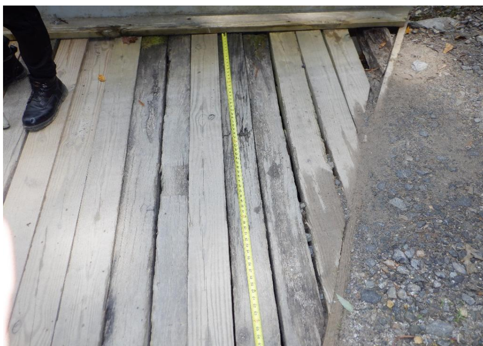
2 DECK BOARDS OVER STR 1/2 DECAYED OVER EB 2
