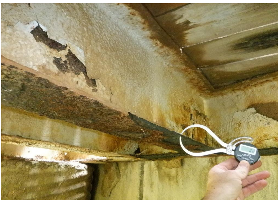
STR 3 BTW FB 1/2- 1/64" REMAINING TO BOTTOM FLANGE 3' SEGMENT
