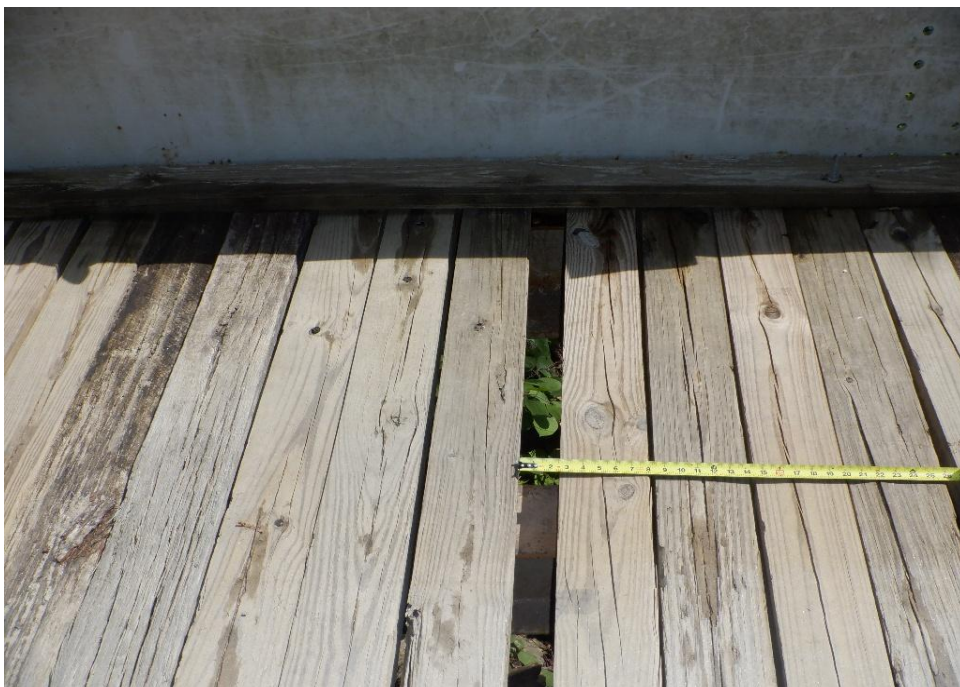
3" GAP IN DECKING BTW FLOORBEAMS 2/3
