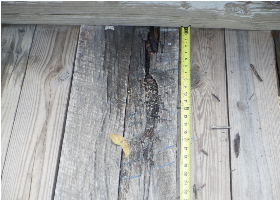
2' X 5.75" AREA OF DECAY IN DECKING N. END AT FLOORBEAM 4
