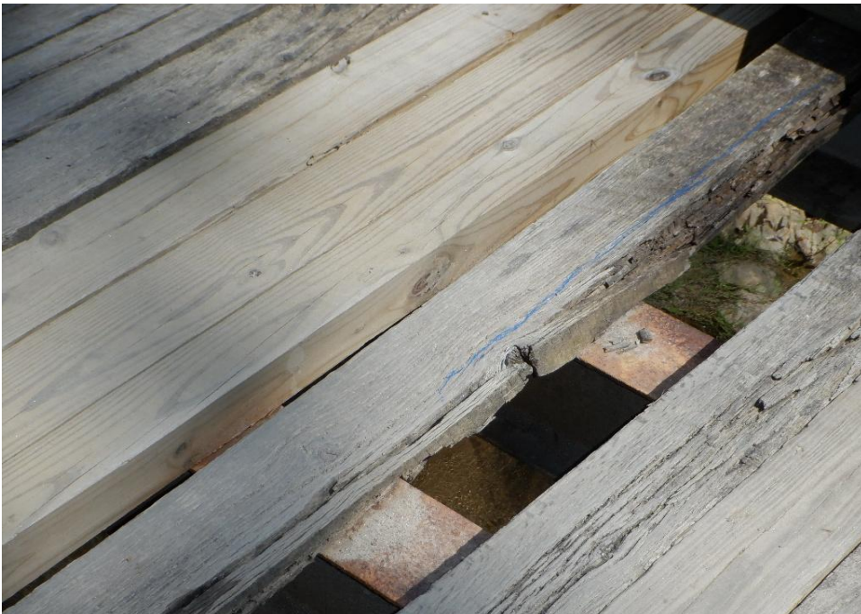
6' L AREA DECAY BTW FLOORBEAM 5/6
